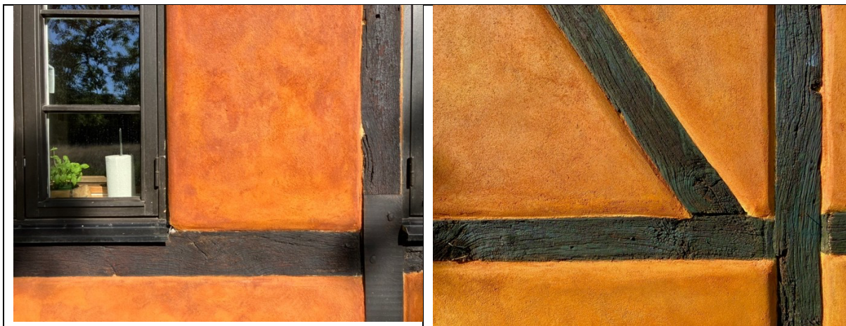
Mixture #F7 applied to fresh lime render. Photographs were taken under different lighting conditions.
